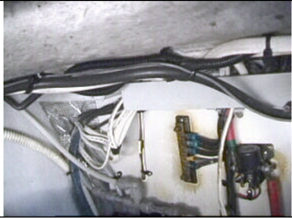
Typical view of electrical wiring support throughout boat.
