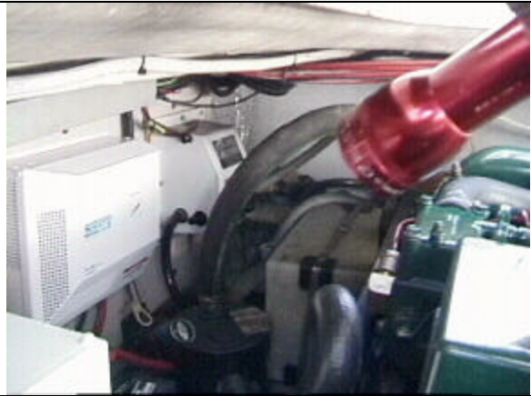
View of forward starboard area in engine compartment. Note Air Conditioning electrical relay box, oil changing box, plastic holding tank.
