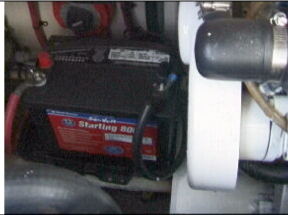
View of forward port area in engine compartment. Note unsecured starting battery for generator. Battery selector switch and single connections to the battery terminal.
